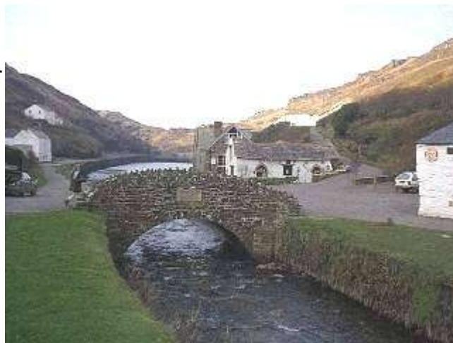
The bridge in the centre of the village, under which debris became lodged, blocking off the channel & increasing the reach of the flood waters
